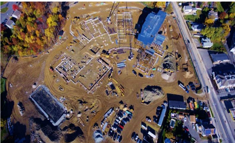
An aerial view of the new middle school construction site from our overhead drone
