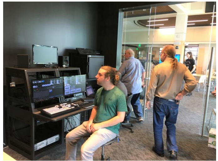
The BevCam staff assisted with the installation of the TV studio at the new Beverly Middle School opening this fall
